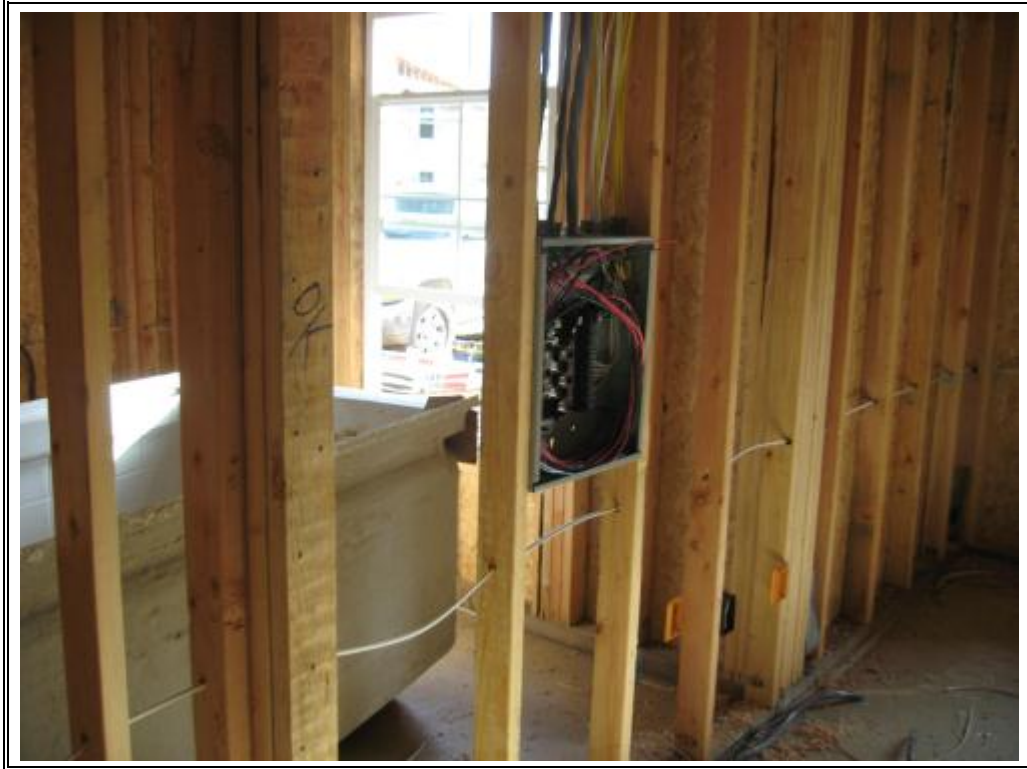
15. Interior unit electrical panel.
