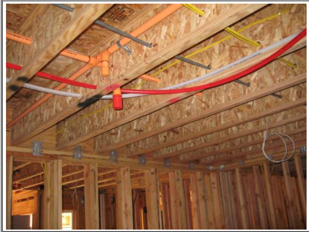
17. Overhead water and sprinkler lines.
