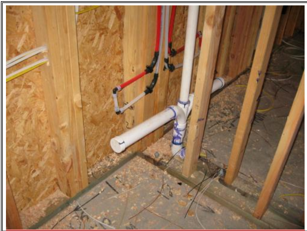
16. Interior lavatory waste and water lines.
