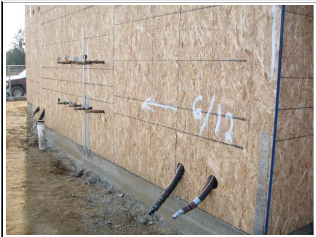
12. HVAC condenser lines and gas meter stubs.
