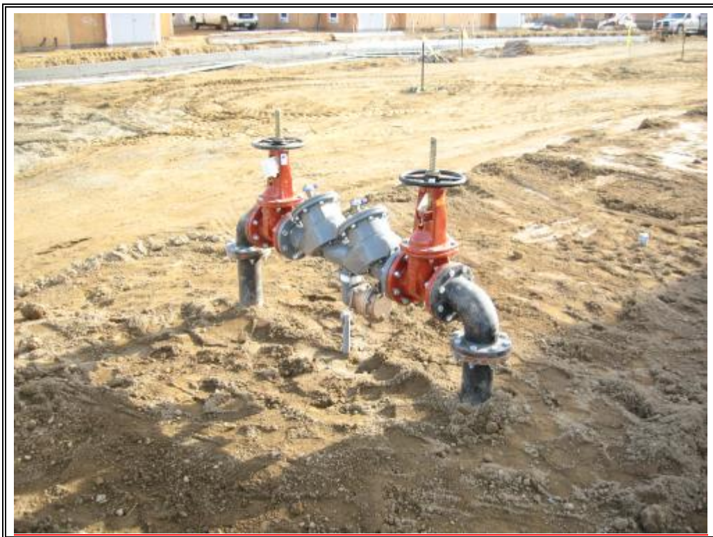
10. Water main valves and backflow.
